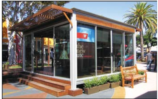
Top: Assembling the hospitality office of the developer at the San Diego Westfield Mall. Aluminum framing members can be designed in almost any rectangular configuration. Post and beam framing allows for larger interior spaces and more glass.
